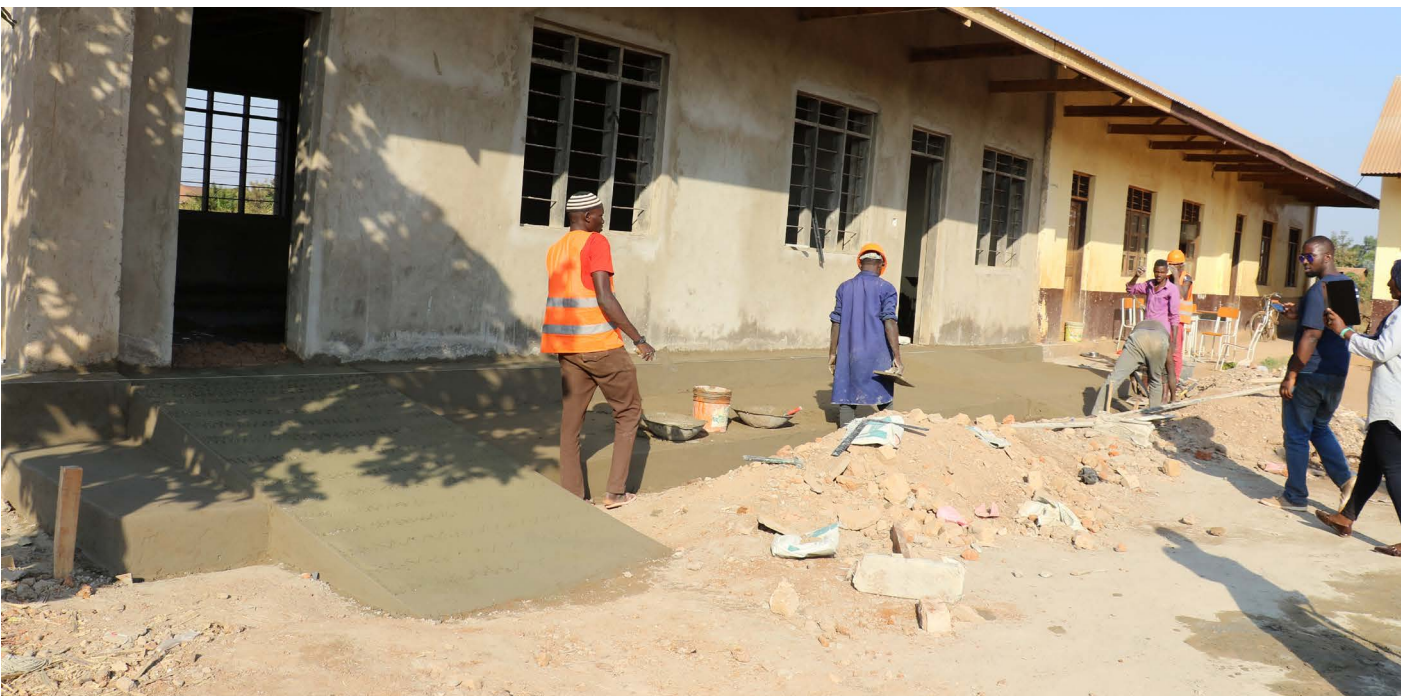
Graduates from a carpentry and masonry classes offered by UNICEF's IPOSA programme working on renovating a government school building. As part of the renovation, they're making the school more easily accessible by persons living with disabilities. IPOSA seeks to benefit youth aged between 14-19 who are out of the formal schooling system through on classes on carpentry, masonry, cookery, decorating, tailoring.
