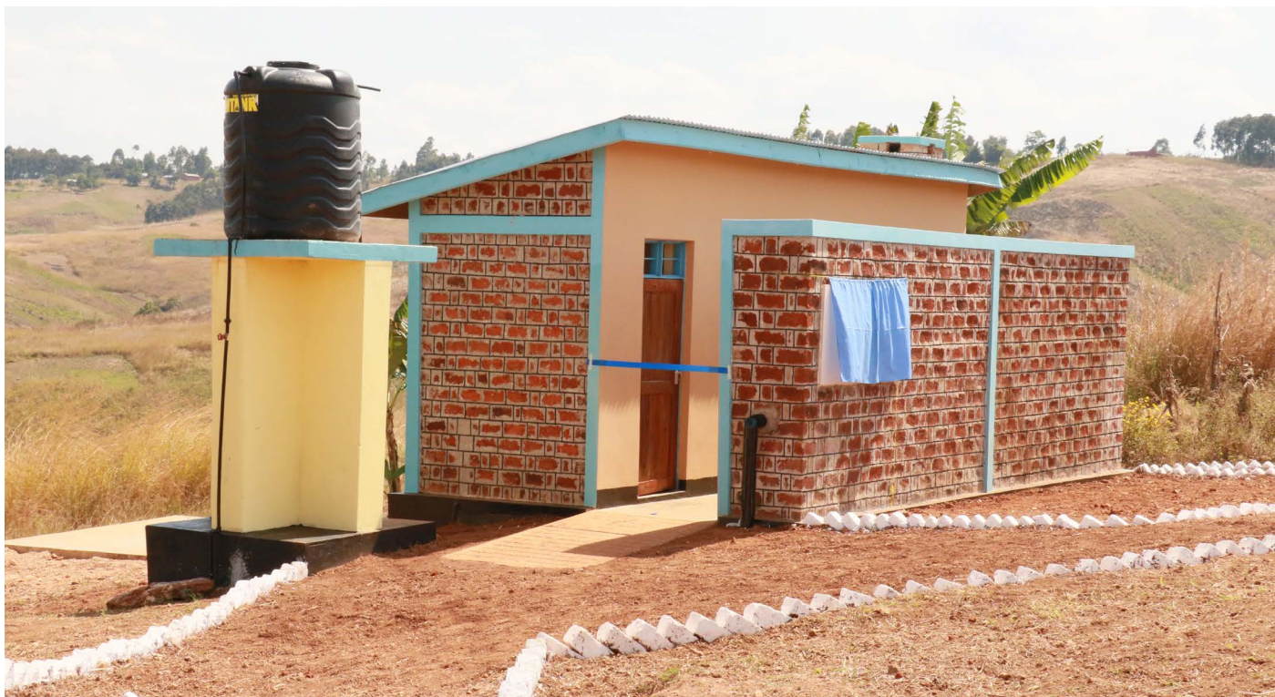
The newly constructed Menstrual Health Management facility at Kumkata Primary School in Kasulu.
