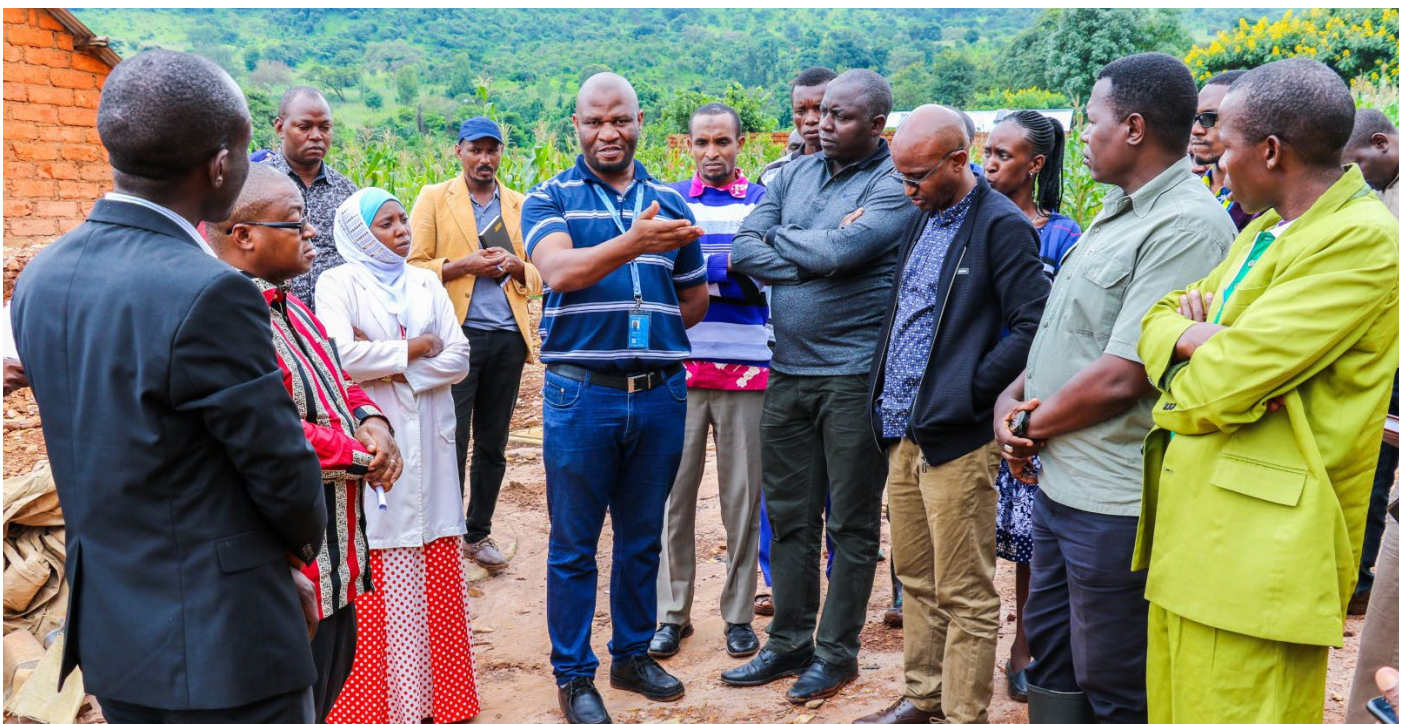
Mr. Evance Siangicha, UN Area Coordinator - Kigoma, briefs the delegation on the ongoing construction of WASH and Health + projects at Kasongati village in Kakonko District.
