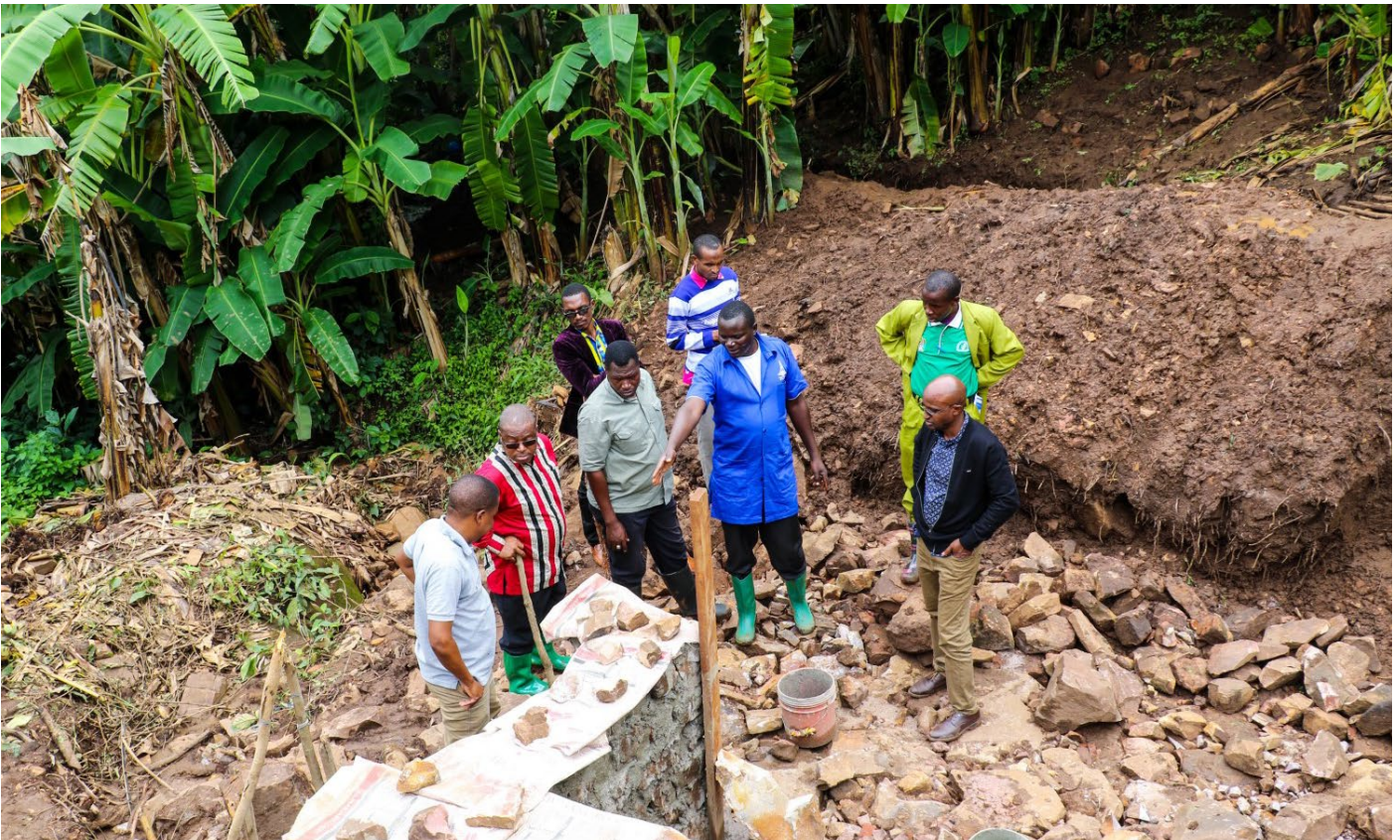
Mr. Rashid Mchatta, Kigoma Regional Administrative Secretary, accompanied by Honorable Hosea Ndagala, Kakonko District Commissioner, and officials from Kakonko district being briefed, by Mr. Emmanuel Busanya TCRS WASH Engineer, on ongoing construction of water intake at Kasongati village. The Project when completed will provide more than 3,075 people with access to improved water service.
