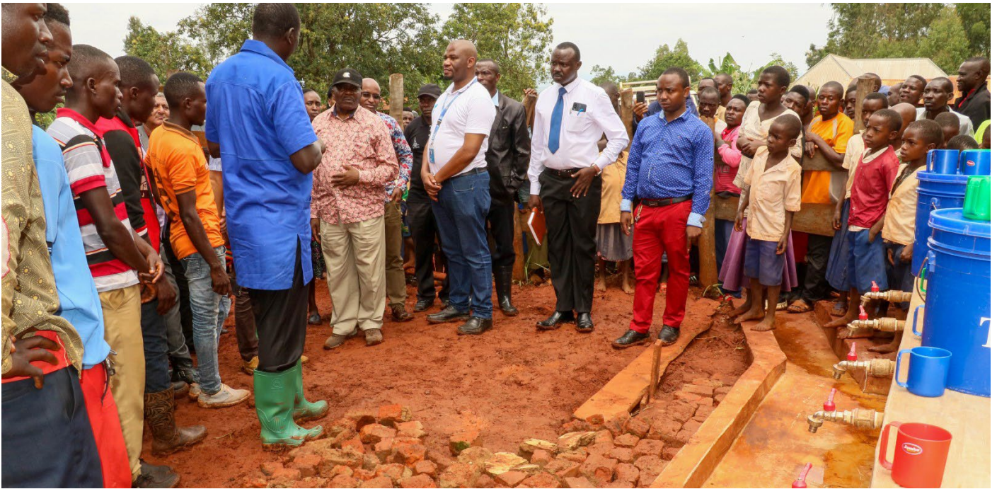
Mr. Emmanuel Busanya (Left), TCRS WASH Engineer, elaborating Kigogo Water Supply System rehabilitation project at the Kigogo Primary School. The intervention has benefited the entire population (about 4,200 people) of Kigogo village including Two primary Schools and One Health Care Facility.
