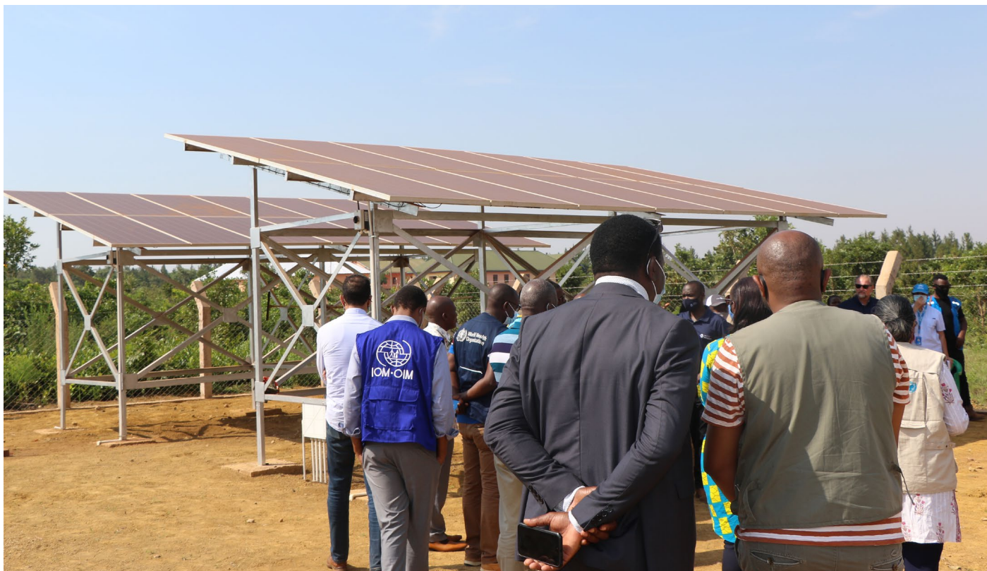
The delegation visited a solarized water supply system which was constructed through the Kigoma Joint Programme (KJP). The water supply system pumps water to Kigoma Grand School in Kasulu District. By providing clean water, the pump has reduced waterborne diseases & improved the students' overall health, attendance & performance at school. © UN Tanzania / Edgar Kiliba
