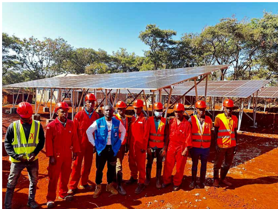
Jupsergi stands with the construction team during installation of the solar panels at the hospital in Nyarugusu Refugee Camp, Tanzania.
