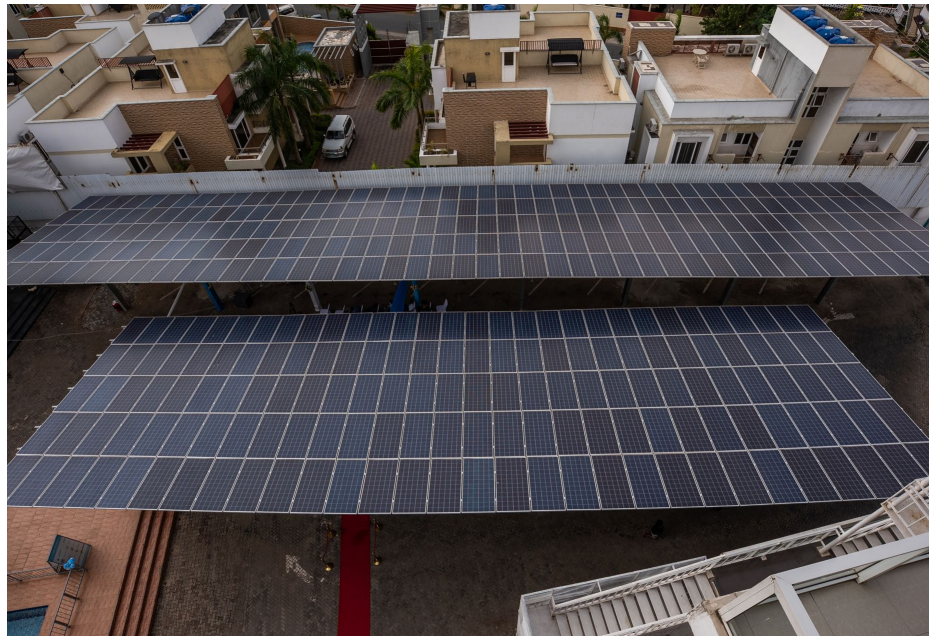
These are some of the hybrid solar panels which are installed at the UN House. The installation of 696 solar panels will generate 70% of power consumption during office hours. Photo | UNDP Tanzania
