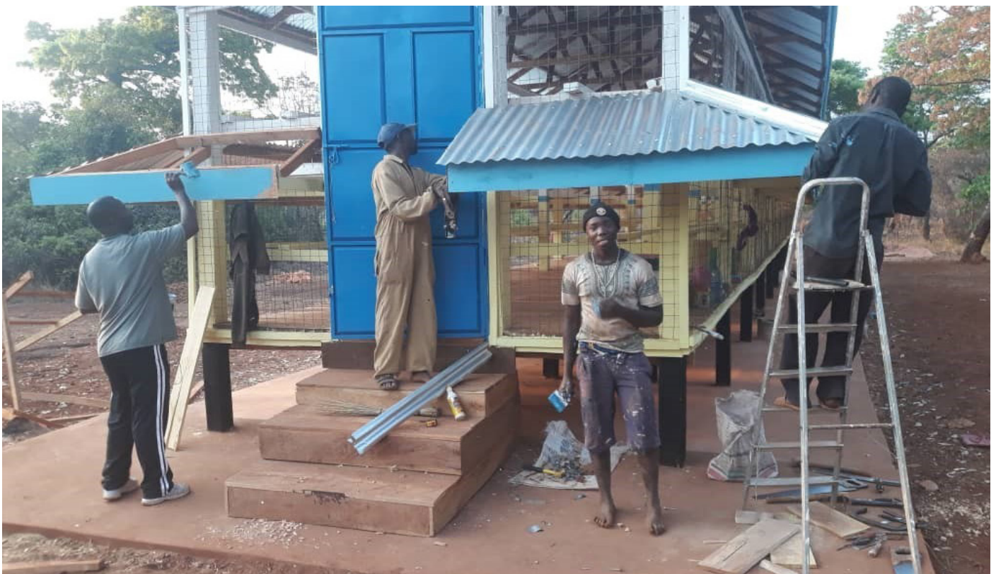
Ongoing construction of the beehouse and beehives by Mr. Hija and his team in the Kibondo District, Kigoma Region. Photo | UN Tanzania
