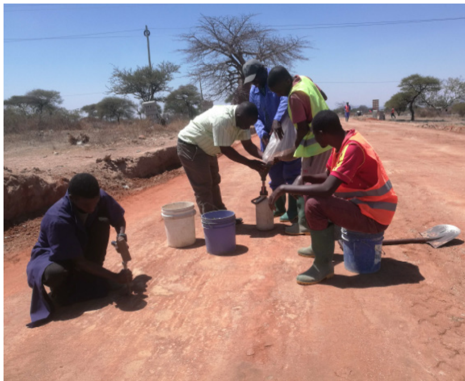
As part of the practical component of the training, participants take part in the laying and compaction of Emulsion Treated Base. Photo | ILO Tanzania
