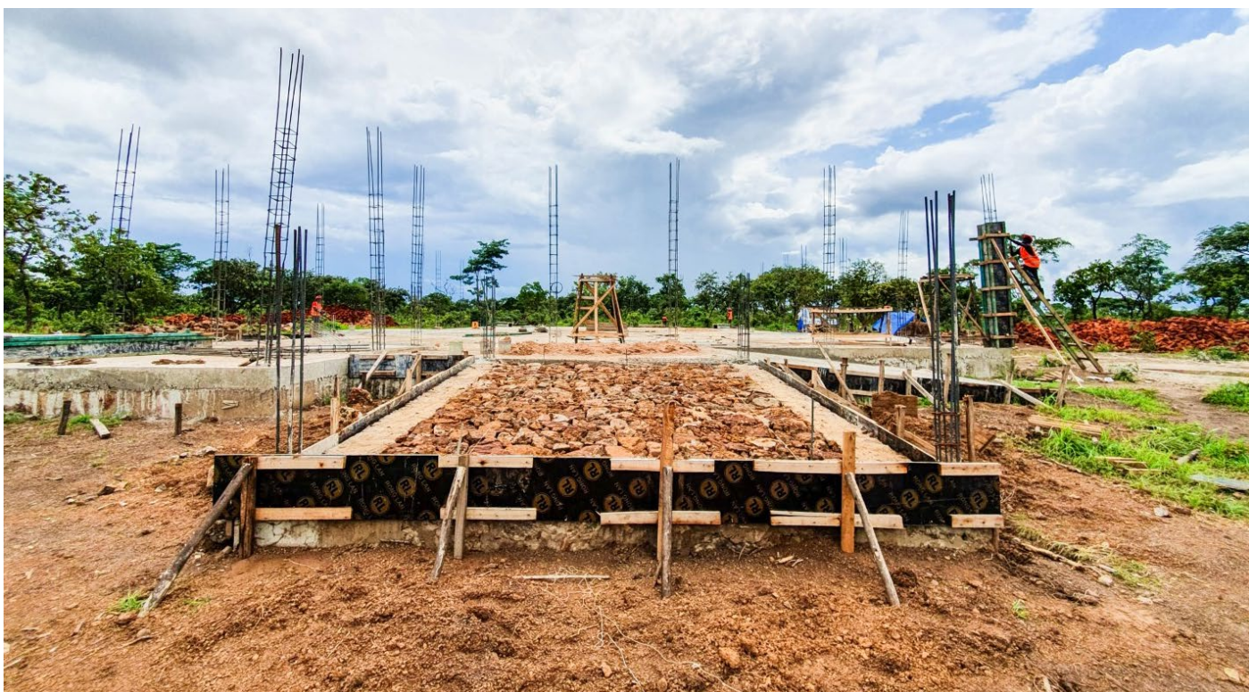
Mvugwe Aggregation Center is currently under construction in Kasulu. Upon completion, the center will provide farmers in the area with proper storage facilities to prevent post-harvest losses and provide market linkages to smallholder farmers.
