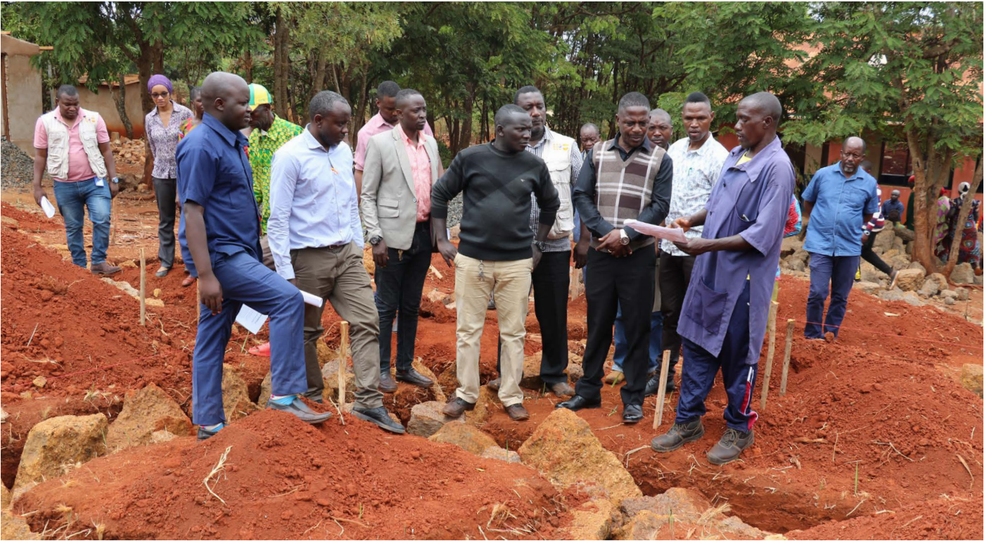
The delegation touring the construction site at Kigondo Dispensary and examining the drawing of the maternity ward to be constructed. The maternity ward will be one of seventeen medical facilities that will be constructed through the KJP of which nine have already been completed.
