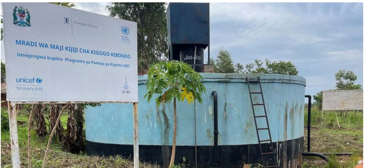
The rehabilitated water storage tank has the storage capacity of 100 cubic meters. The tank supplies water to the Kigogo community of 4,232 residents.
